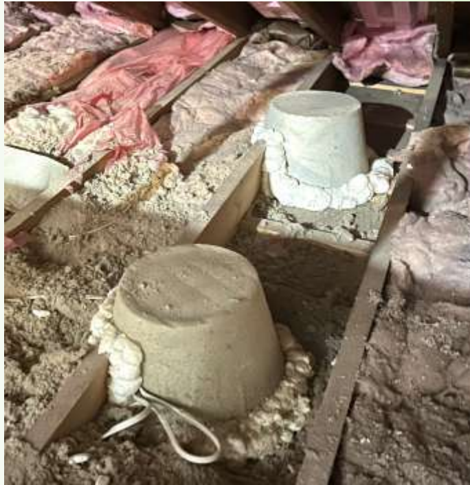
"Can covers" over recessed lights
