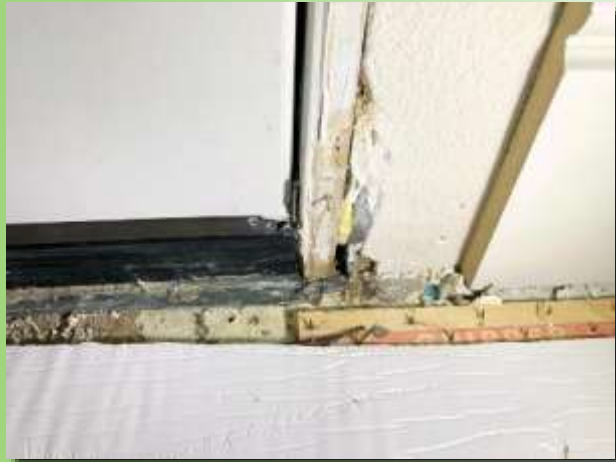
Cracks around exterior doors
