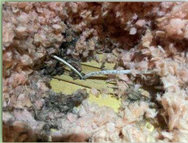
Pipe & electrical penetrations
