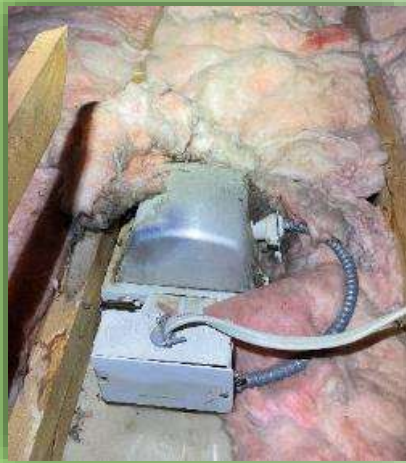
Ceiling lights & bath fans
