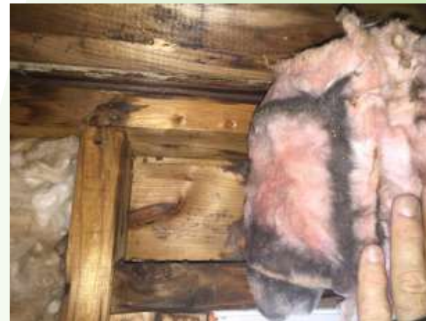
Stained “filter-glass” from air leakage
