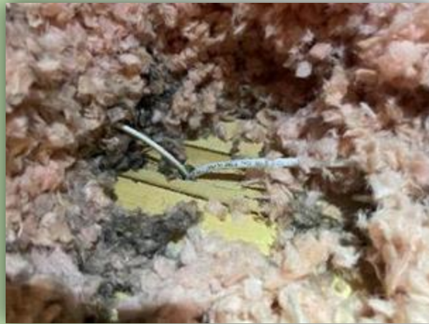
Pipe & electrical penetrations
