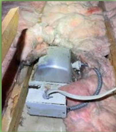
Ceiling lights & bath fans
