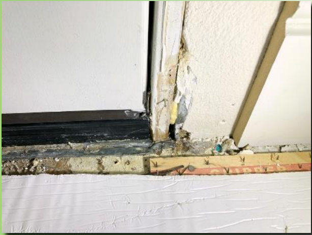
Cracks around exterior doors
