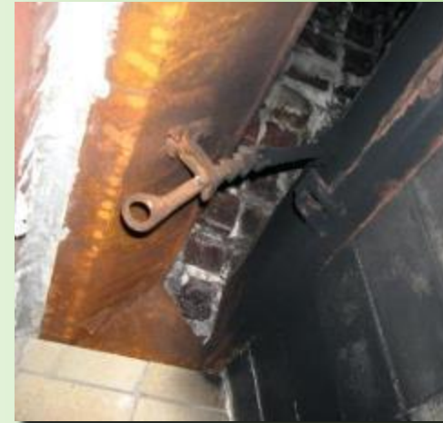
Fireplace & woodstove flues
