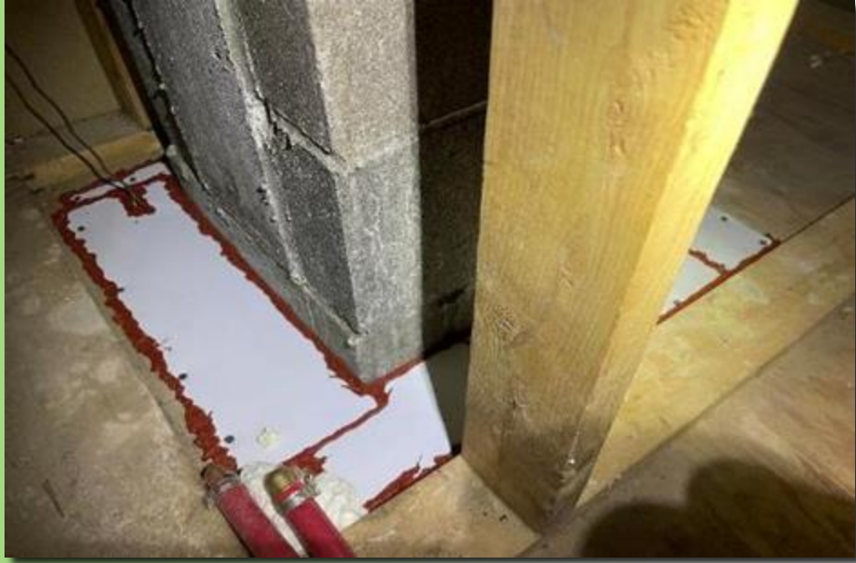
Air sealed chimney chase w- fire-rated materials
