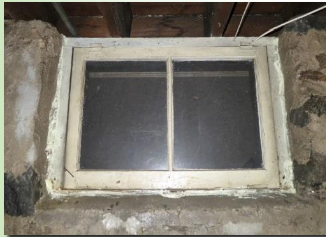
Around old basement windows
