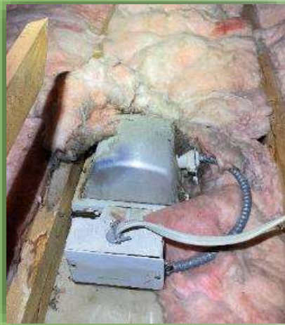
Ceiling lights & bath fans
