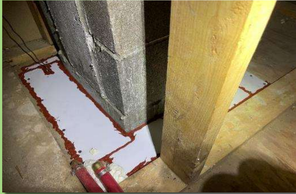
Air sealed chimney chase w- fire-rated materials
