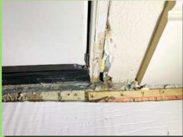
Cracks around exterior doors
