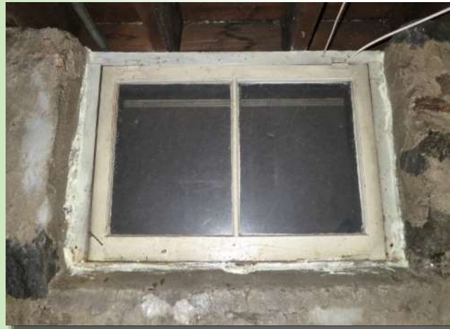
Around old basement windows
